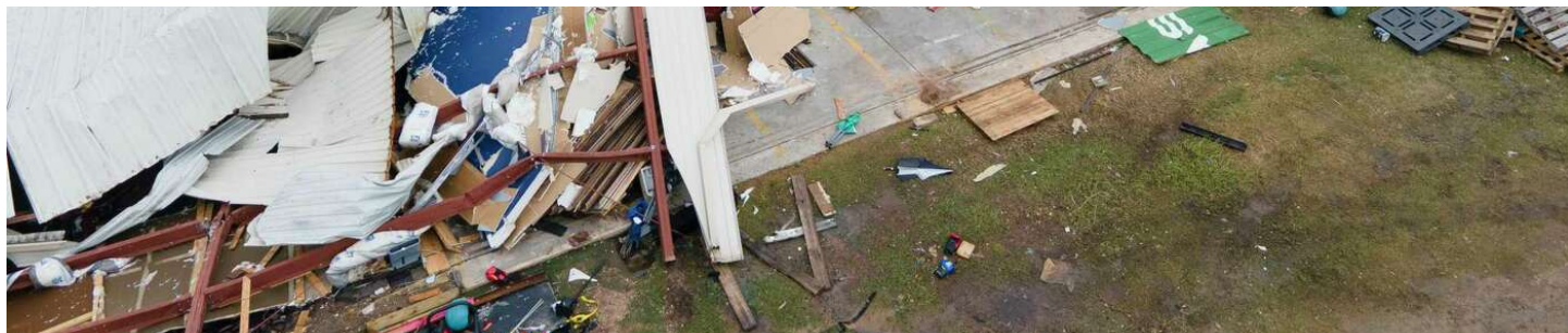
Damage to the IsoKinetic Speed Development building along Pansy Street is seen from Tuesday's tornado that touchdown down, Wednesday, Jan. 25, 2023, in Pasadena.
