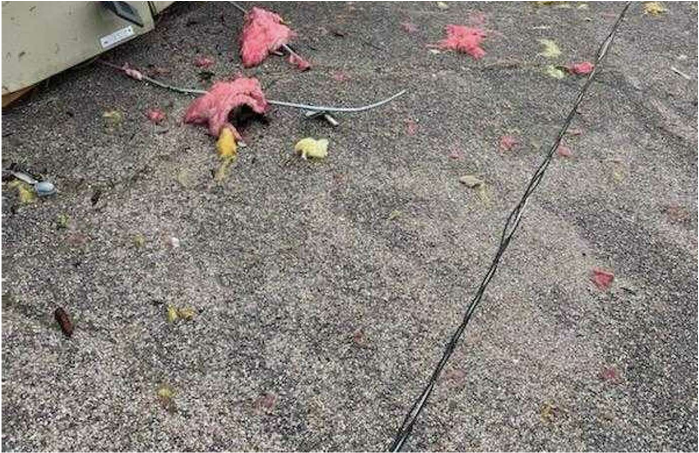
A portable building at Teague Elementary on Burke Rd. in Pasadena was damaged in the storm. (Yvette Orozco)
